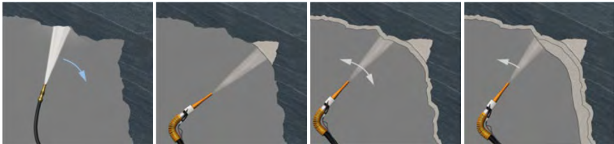
Figure 65: Steps in shotcrete practice: (from left to right) 1. Cleaning using high pressure water; 2. Filling of overbreak; 3. 1 st shotcrete layer (excavation stabilisation and adhesive bridge for second layer); 2 nd shotcrete layer (excavation stabilisation) usually together with steel reinforcement (e.g. mesh) (Lindlar et al. 2020)
