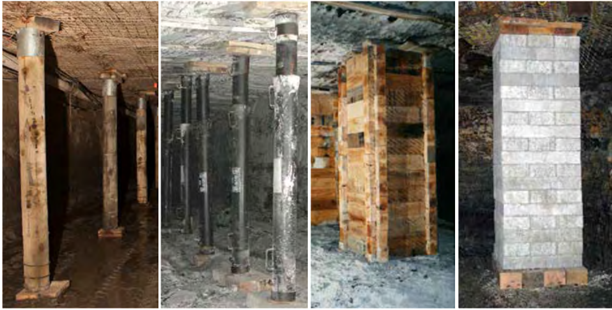
Figure 57: Strata Worldwide secondary roof support: (from left to right) Timber standing prop support; (active) steel props; timber crib support using stacked interlocking blocks; concrete crib support using fibre reinforced blocks ( www.strataworldwide.com/mining/strata-geotech-mining/roof-support-mining )
