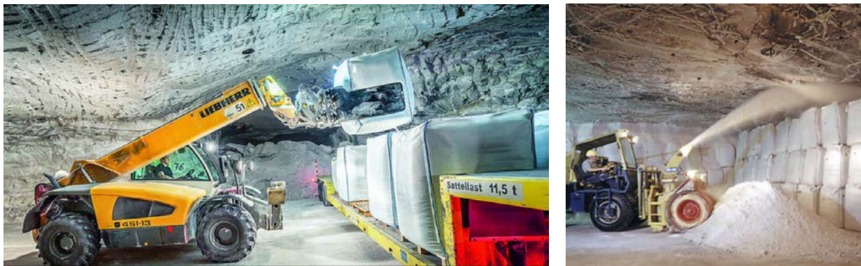
Figure 7.3: Mechanical backfill methods: Big-Bag backfill and slinger backfill method in practice in the K+S mines in Central German (Pictures REKS GmbH & Co. KG, formerly K+S Entsorgung GmbH, Kassel, Germany).
